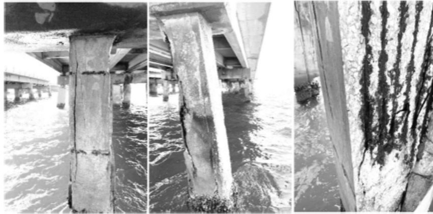
Fig. 17—Corrosion progression in prestressed piles: (left) corner cracks; (center) corner spalling; and (right) cover loss (courtesy of FDOT).
