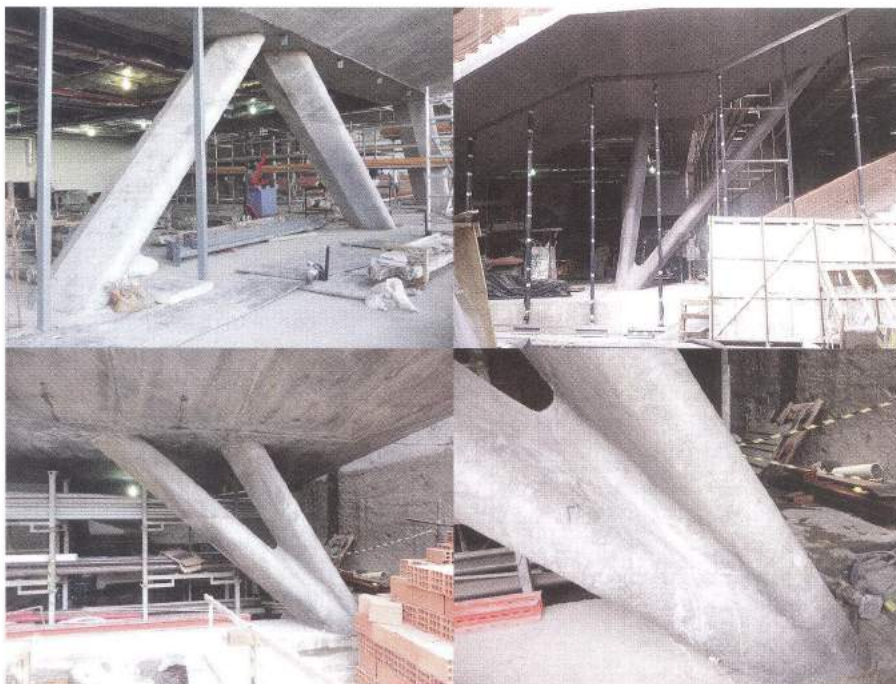
Fig. 6: Actual inclined columns in the building exhibit the high-quality finishes required of the exposed structural and architectural elements
