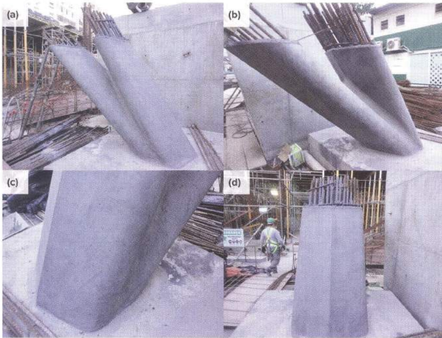
Fig. 5: Mockup finishes: (a) sides; (b) sides and lower region at joint; (c) detail at base and joint; and (d) overview of upper inclined region
