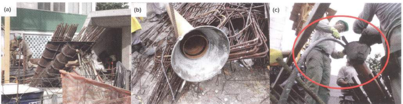
Fig. 4: Casting the inclined column mockup helped in the evaluation of various factors: (a) metal forms and inclined reinforcement projected from a previously cast base joint; (b) a drop tube was used to deliver concrete from the concrete bucket to the base of the column form; and (c) a bottomless pail acted as a funnel and reservoir for concrete, allowing a vibrator to be inserted into the drop tube without overflow
